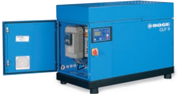
The frequency converter with its built in control is integrated neatly into the existing electrical cabinet.
